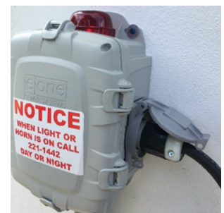
Generator Cord Connected
