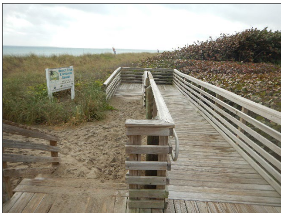
Image 10 Boardwalk ramp at Jensen Beach covered by sand.
